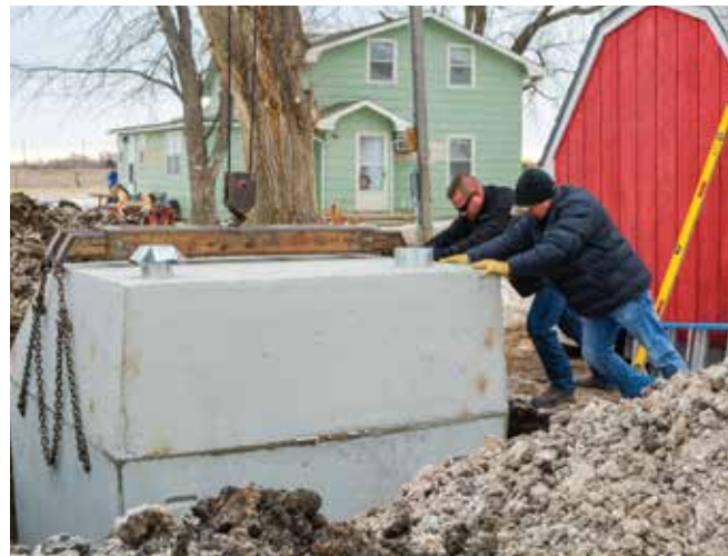
Eric Stolfi and Jesse Kutleck install a storm shelter for Flint Hills Electric Cooperative member Nick Williams.
